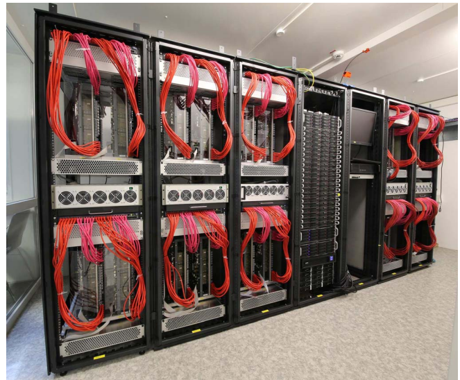
Fig. 1. The BrainScaleS system as it is currently installed consisting of five cabinets, each containing four neuromorphic wafer-scale systems. Upstream connectivity to the control cluster is provided by the prominent red cables, each communicating at Gigabit speed. This enables fast system configuration and high-throughput spike in- and output. An additional rack hosts the support infrastructure comprising power supplies, servers, the control cluster, and network equipment.
